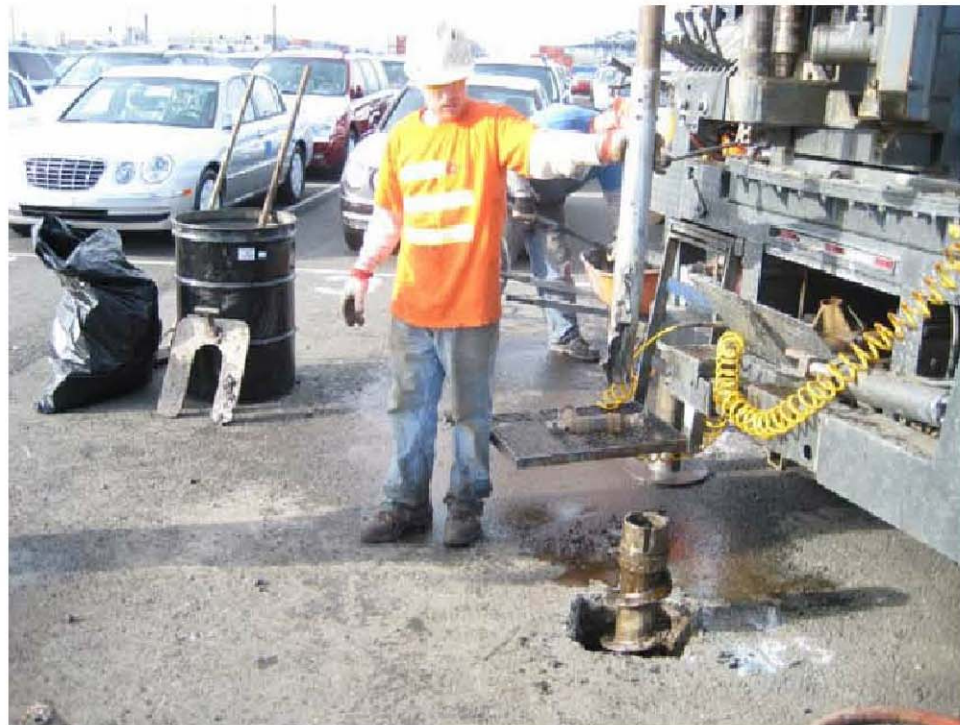
Photo 3. Core sampler damaged by subsurface rocks.
